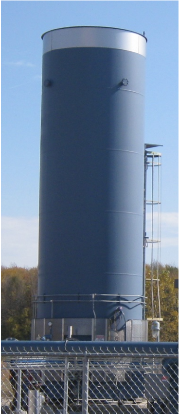
Enclosed Flare (re-tool? supp. fuel?)
