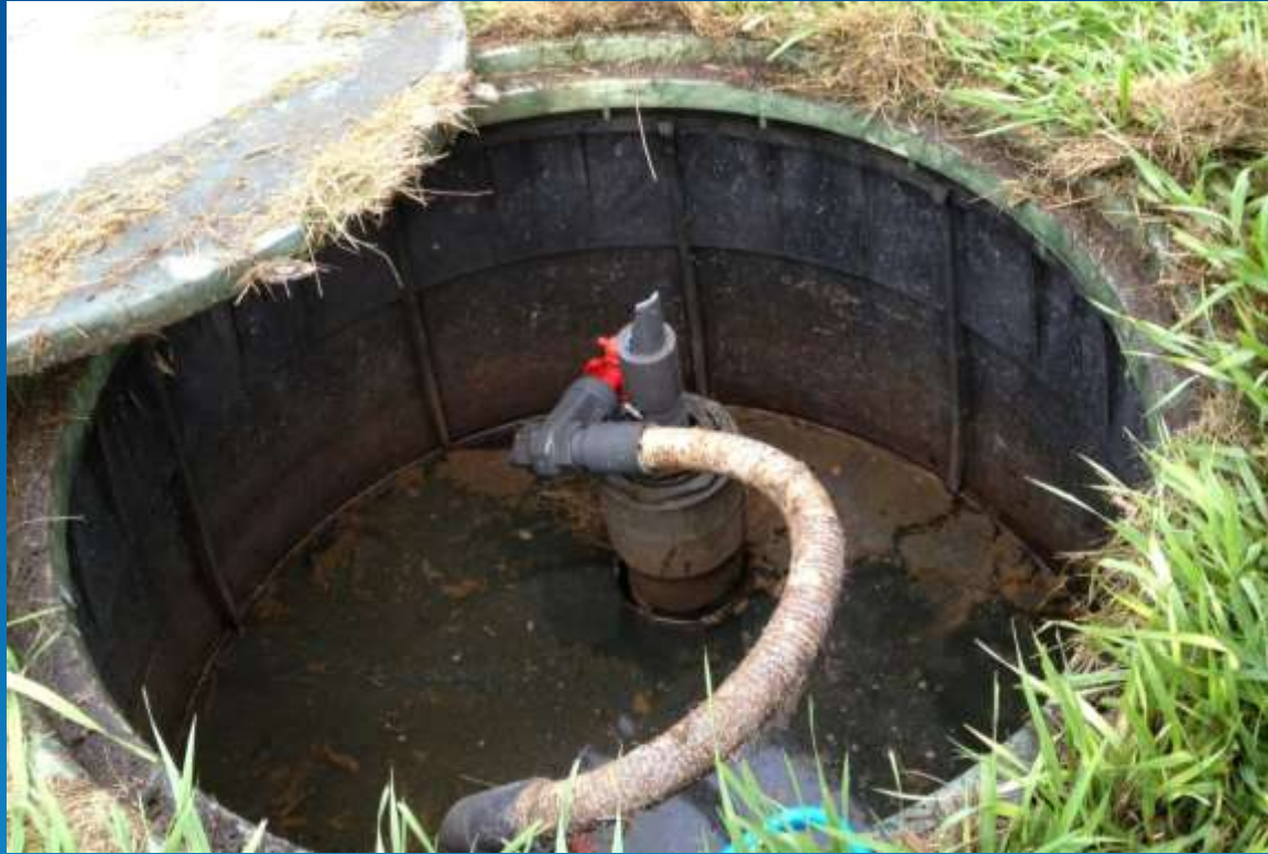
Wellhead Damage Flooding
