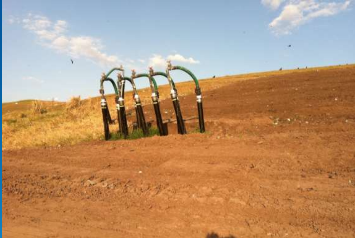
Typical Above Ground LFG Wellheads
